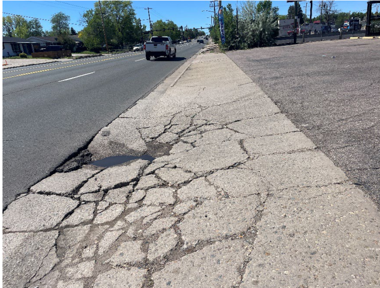
Figure 9. Segment of sidewalk in disrepair between Jewell Avenue and Evans Avenue.
